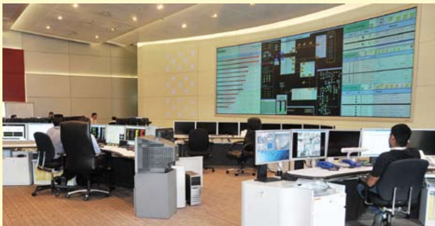
TNB's National Load Despatch Center
